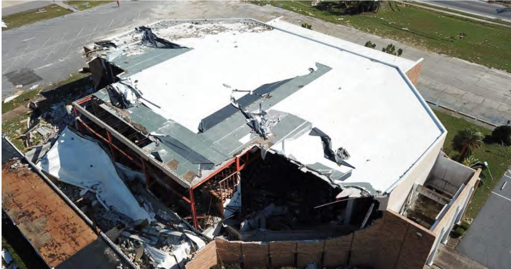
Wind Uplift failure. Image courtesy of StEER.
