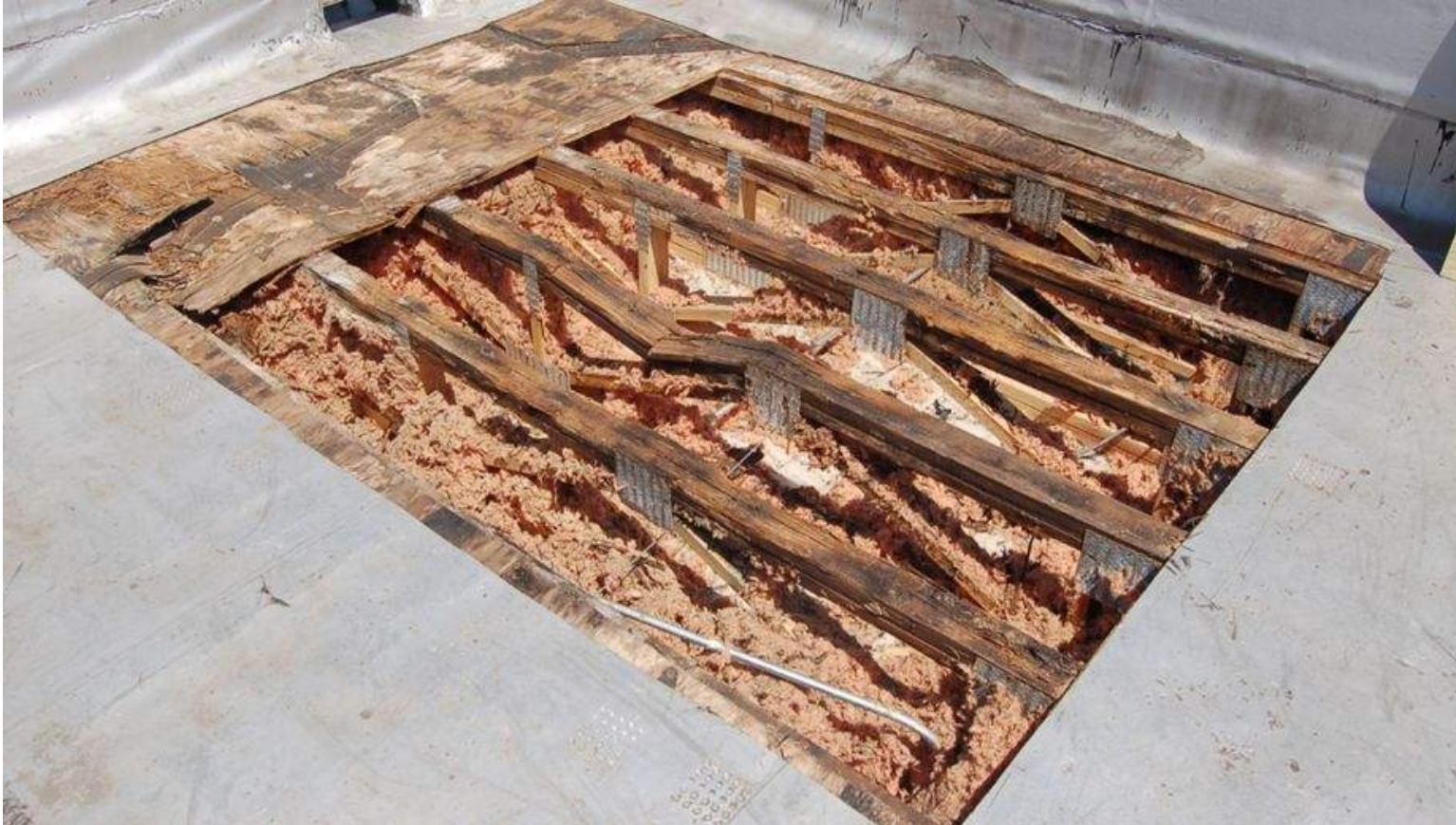
Commercial roof failure. Image courtesy of Phil Dregger.
