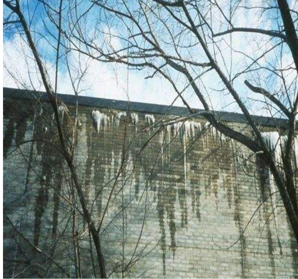
Commercial building failure at parapet. Image courtesy of Intertek
