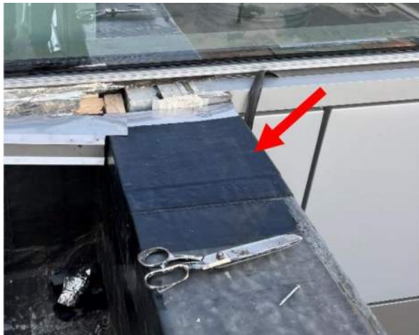
Figure 9.1d – Uncured EPDM used to transition from existing EPDM at parapet onto stainless steel saddle.
