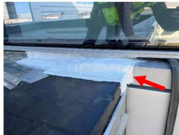
Figure 9.1e – Silicone transition sheet (boot) installed from stainless steel saddle flashing to primary sealant below window. Silicone extends only 1/2" onto existing metal panel (red arrow), in order to be concealed by parapet fascia.
