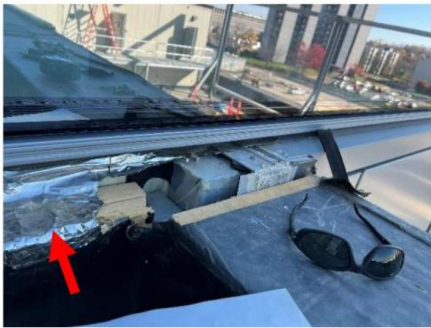
Figure 9.1a – Parapet to building wall transition. Red arrow points to York flashing, which laps over EPDM at vertical wall.
