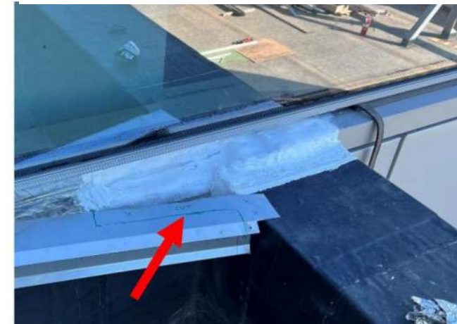
Figure 9.1f – Silicone transition sheet (boot) installed. Existing counterflashing identified to be cutback (red arrow) so as not to damage silicone boot when installed.
