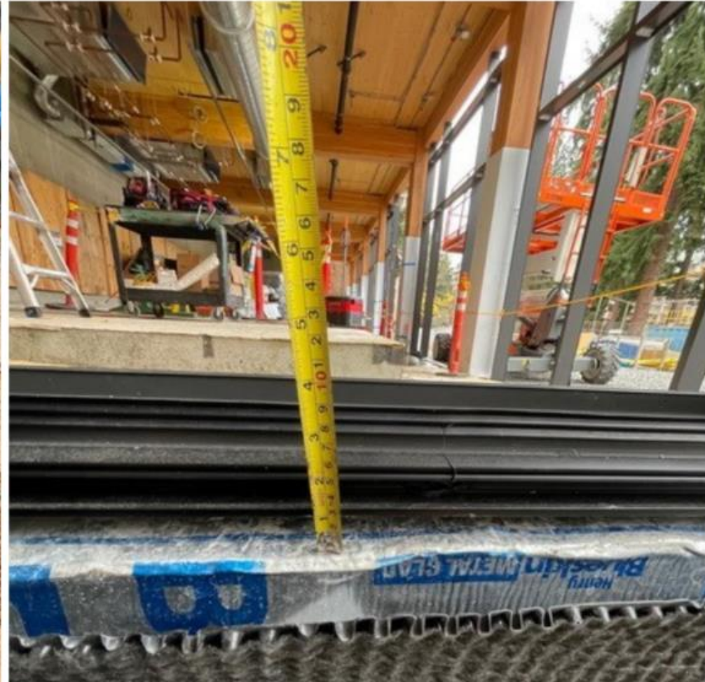
SV.07.02.D - The gap between the horizontal mullion and the concrete surface was measured at 3/4".
