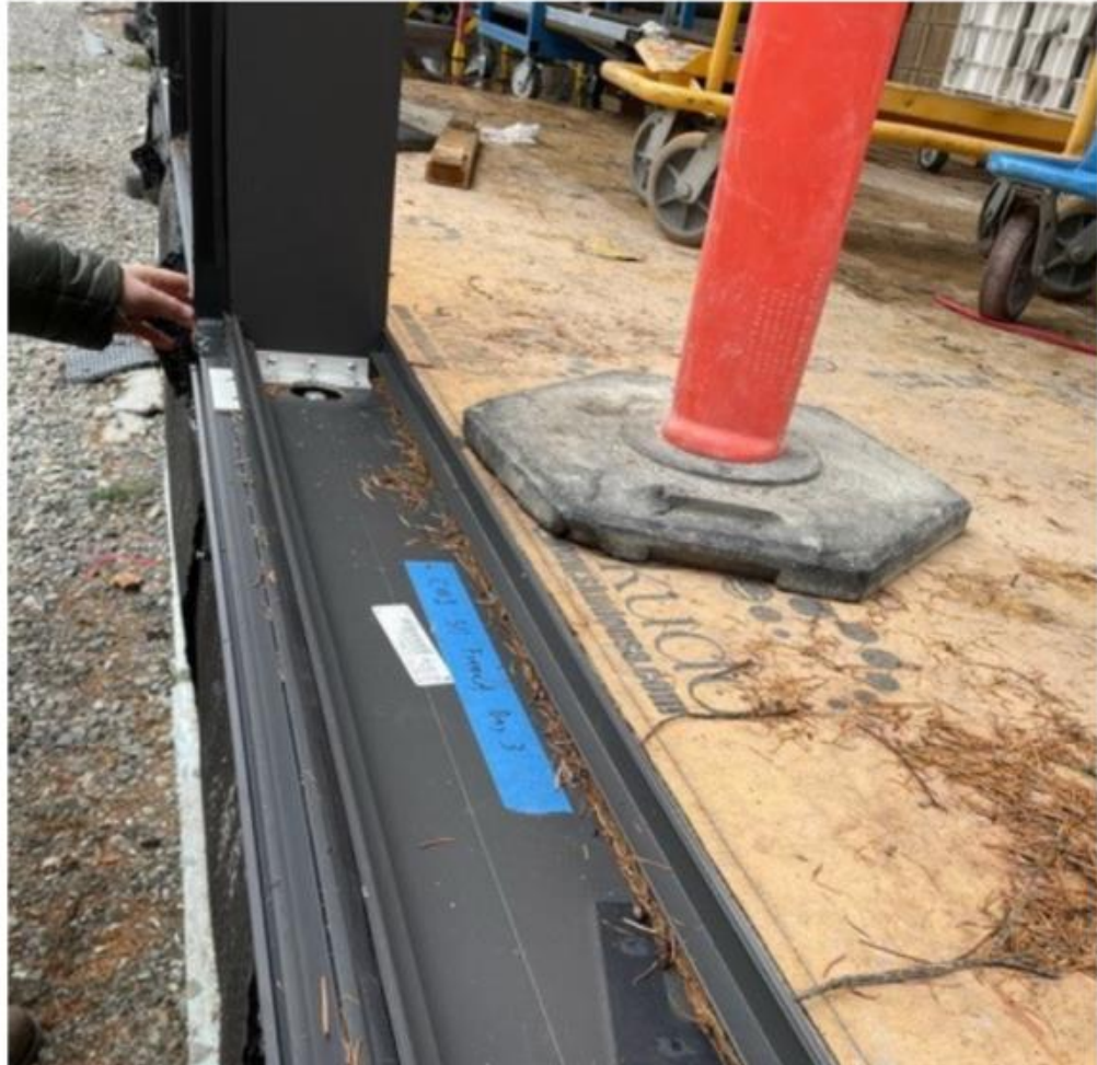
SV.07.02.C - The setting blocks had been placed at the curtain wall sill.
