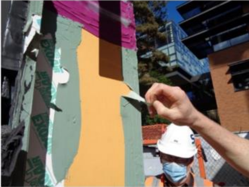
SV.01.02.D - MH observed insufficient adhesion between Dymonic 100 and ExoAir 430 panel.
