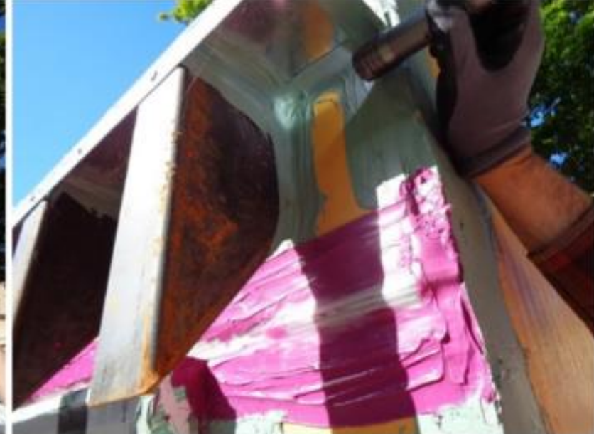
SV.01.02.F - MH observed multiple holes at one knife through tooled sealant.
