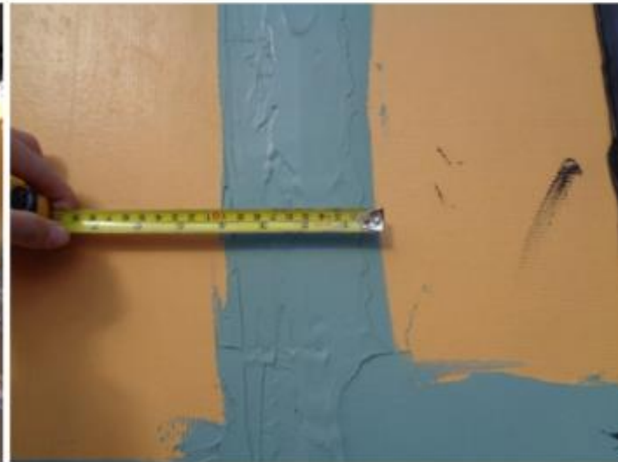
SV.01.02.B - Sheathing joint tooled with Dymonic 100. A min. 3/4" sealant was measured at each
