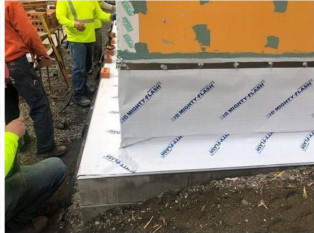
SV.05.02.B - Thru wall flashing installed over base of wall flashing. Termination bar installed at top of thru-wall flashing.
