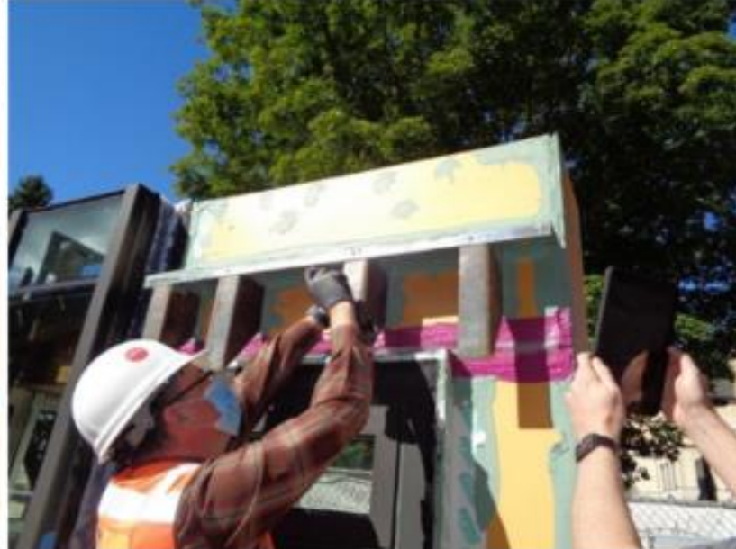
SV.01.02.E - View of tooled sealant around the knife penetrations on the sheathing.
