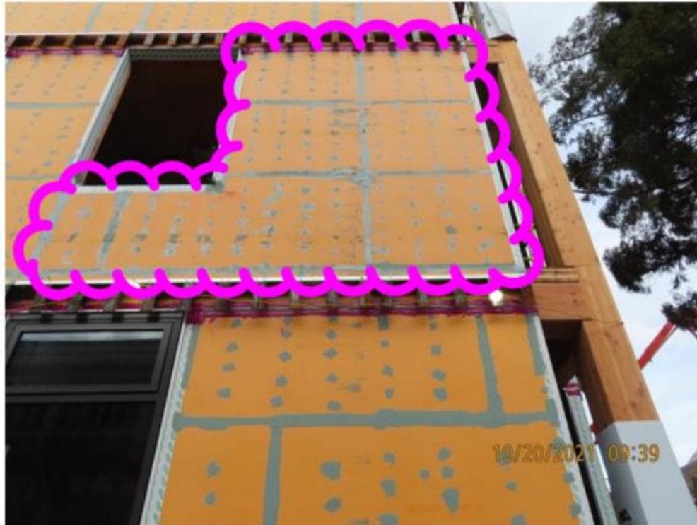
SV.05.01.C - Sealant over fastener heads appears abraded.
