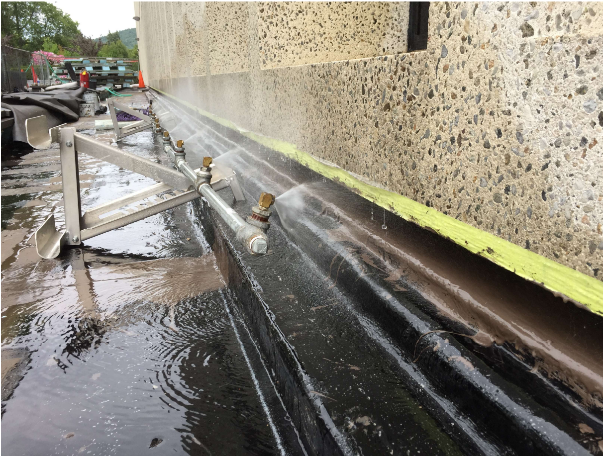
Spray rack testing
