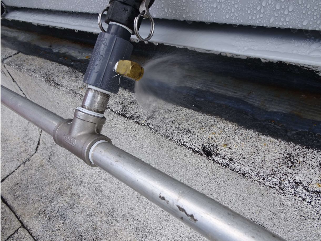
Spray rack testing
